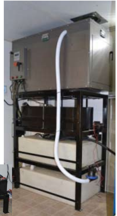
Rack with Waste Combustion System and Tanks
